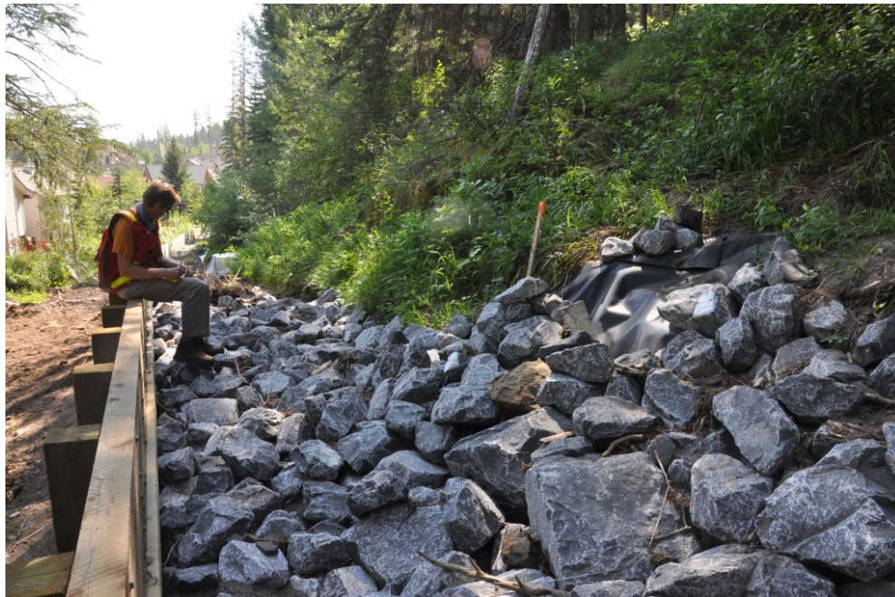
Photo 4-2. Lined and riprapped interception channel on Y Creek above Wilson Way. The riprap and liner were placed following the July 2012 storm. BGC photograph of July 25, 2013.
