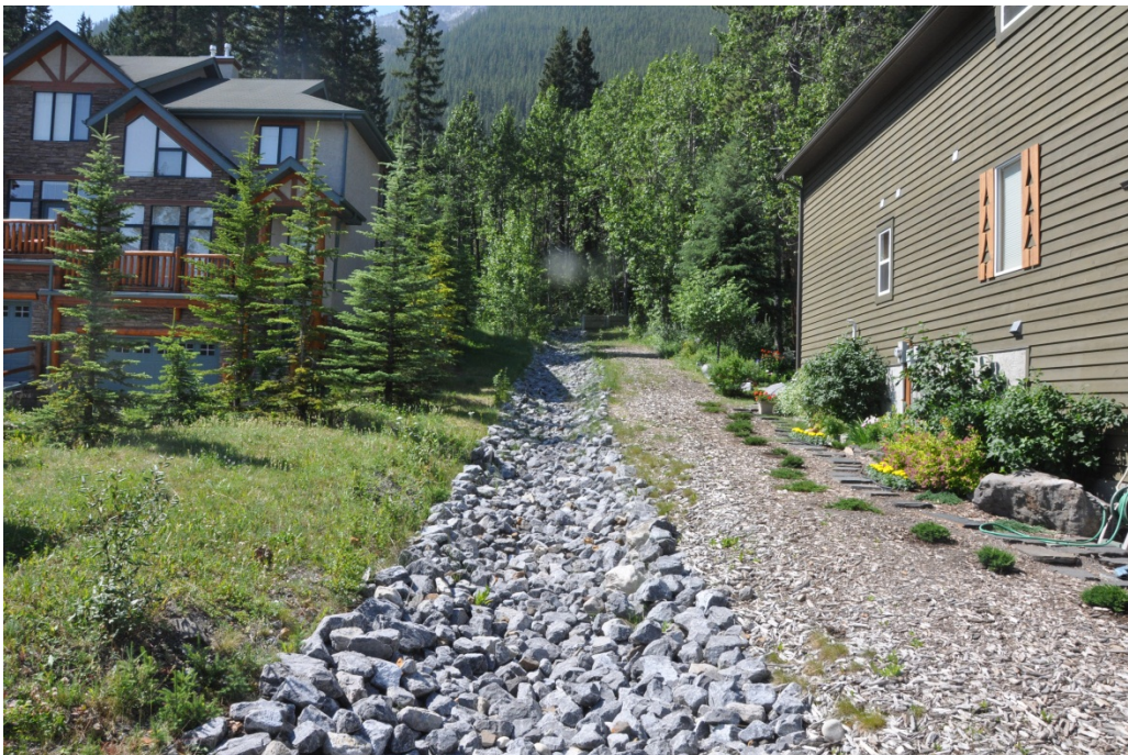
Photo 4-5. Upstream view of riprapped channel installed downstream of the V-shaped wooden wall shown on Photo 4-4. BGC photograph of July 25, 2013.
