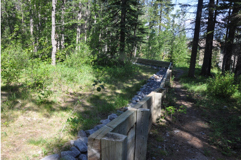
Photo 4-4. V-shaped, deflection wall installed upstream of development on Wilson Way. This structure is located along Y Creek, although no identifiable channel was observed upslope of the wall. BGC photograph of July 25, 2013.
